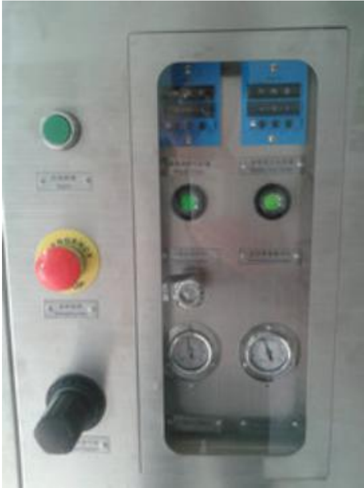
New control panel
